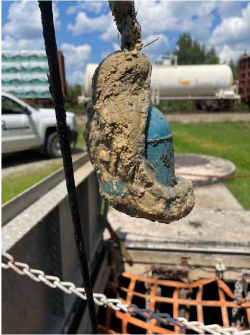
A float partially covered in grease.
